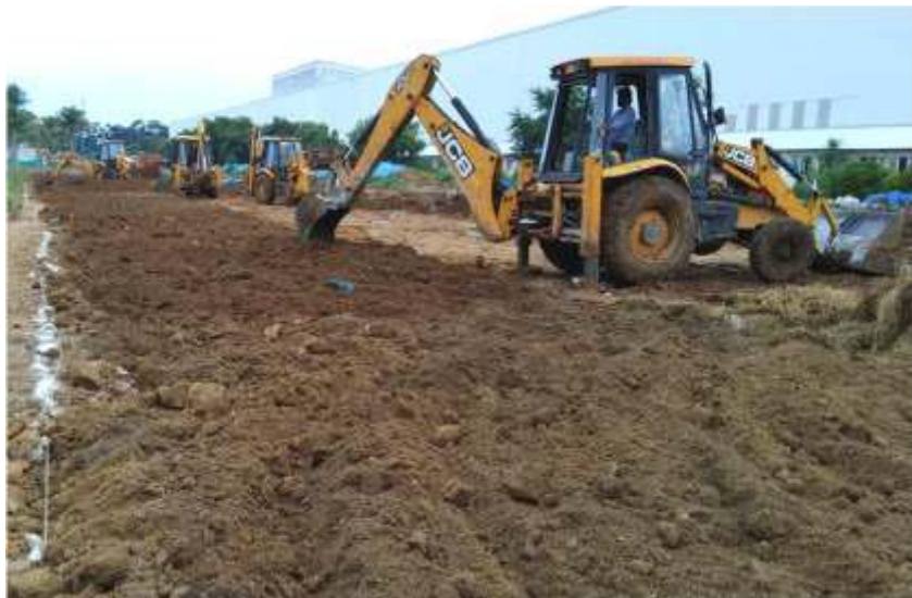
Thoroughly mixing the biomass with the soil beneath 2 feet using the machine
