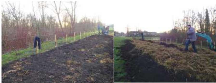
Above: Dumping remaining half of the soil into the pit and spreading the remaining biomass on top of the soil
