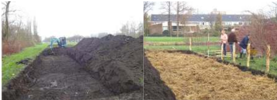
Above: Excavation or 1 meter trench digging, dumping back half the soil, spreading half of the biomass, then followed by mixing
